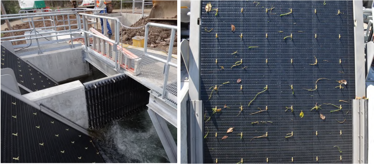
Figure 4-17 - Photos of the North Fork TSS Traveling Screens with Debris Pegs
