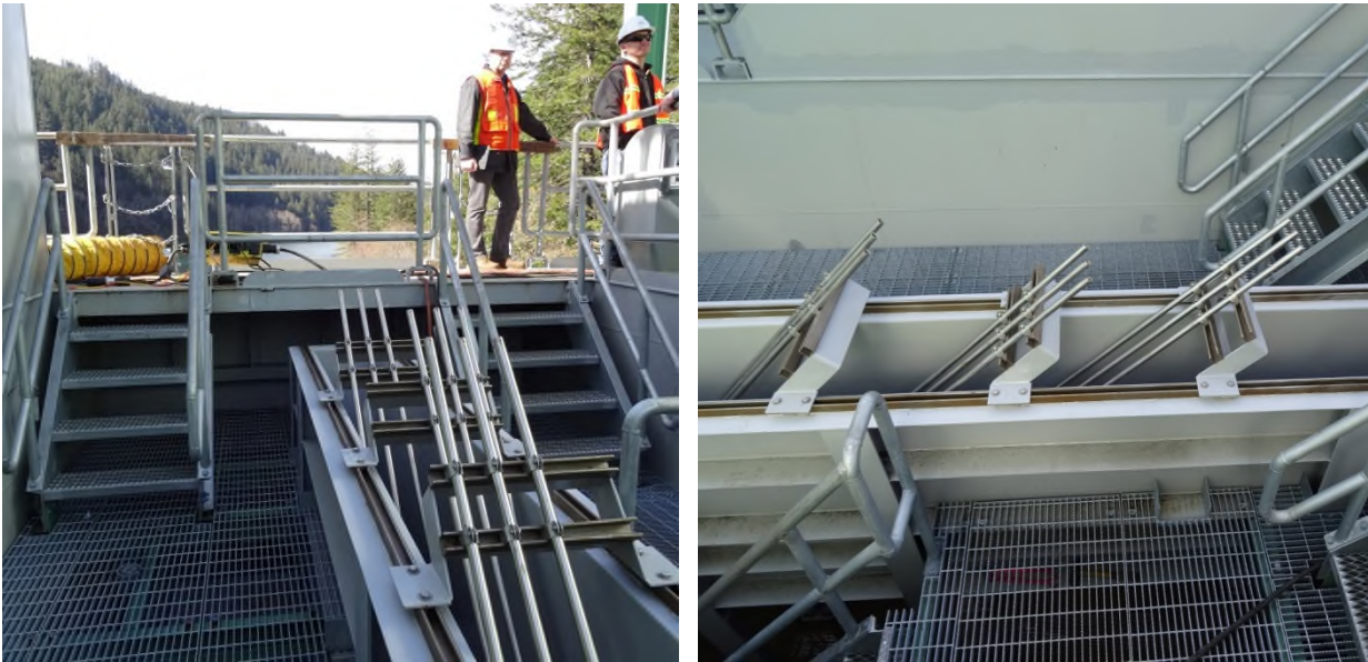
Figure 4-15 - Photos of the Debris Rack in the North Fork FSC Transport Flume
